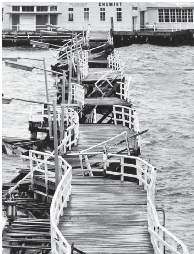
Storm damage to Manly promenade, Sydney 1974.
