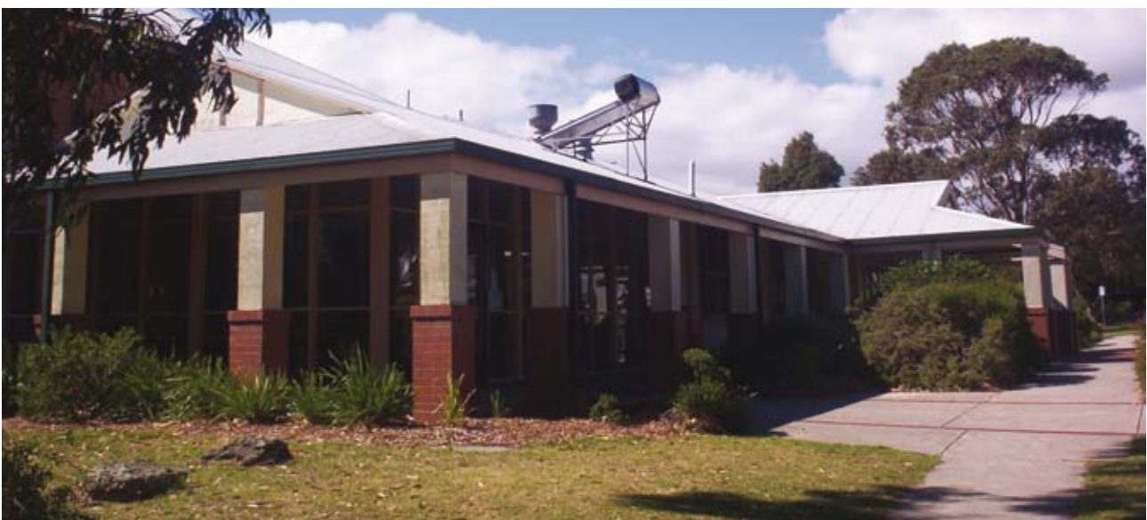
Solar hot water panel – Bass Coast Shire Civic Centre Photo Courtesy: Western Port Greenhouse Alliance
