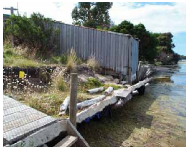
Eroding soft rock shore (clayey gravels) at Anson's Bay, north east Tasmania. The photo (2002) shows a poorly constructed ‘coastal defence’ that is collapsing because of undermining of the shore in front.
